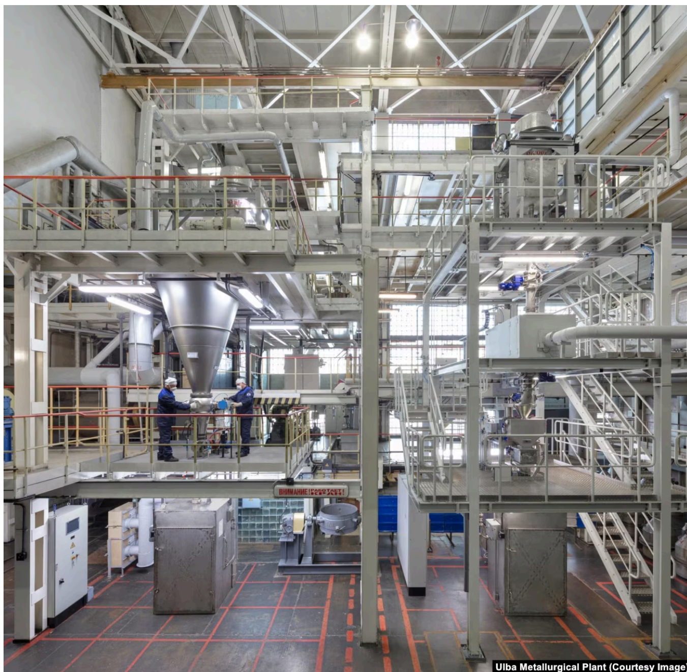
Ulba Metallurgical Plant (Courtesy Image)
